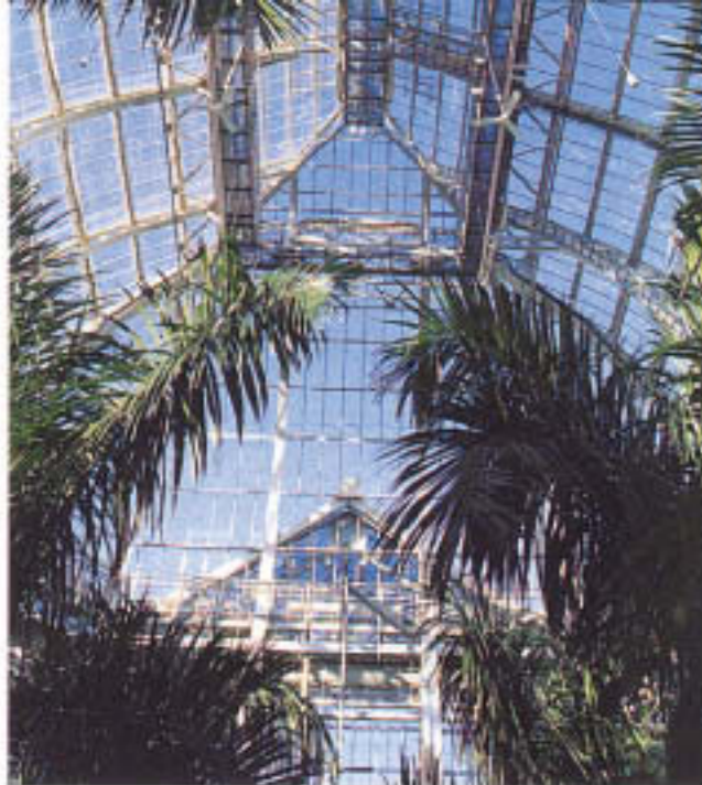
Left: More than 20,000 panes of glass were installed in the conservatory. Shown here is the Palm House.
